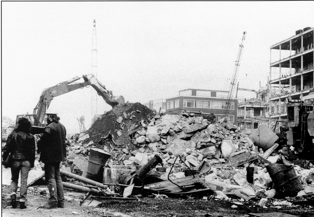
Demolition of Player's 1932 extension. Photo by Brian Thomas, courtesy of Local Studies Library, Nottingham Central Library. Information from Radford Library: Demolition of Player's premises where the shopping complex now stands took place 1984-87. The extension clock was reused in the shopping complex.
